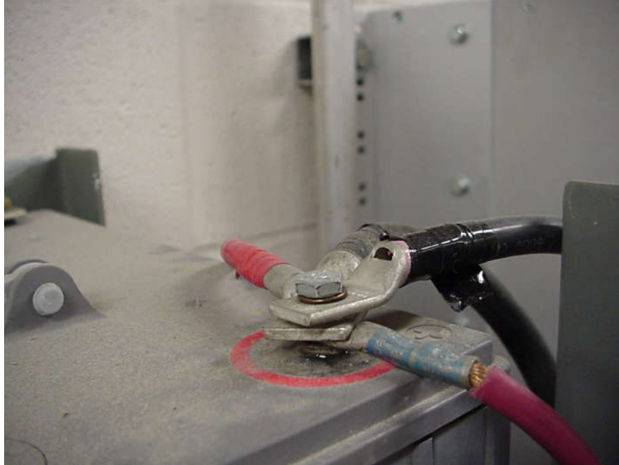
Figure 1. Battery terminals should not be the center point of a DC system!
